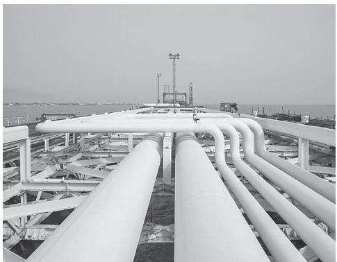
The managing Director of Iranian Oil Terminals Company (IOTC) has said his company is accelerating its currently underway development projects in the country's oil terminals in order to be fully prepared
